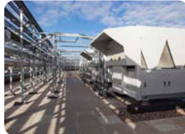
Prince Charles Hospital Electrical, LTHW, CHW £49.0m (M&E)
