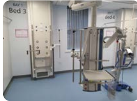
Bradford Hospital Wards 10, 2 and 5 £3.6m (M&E)
