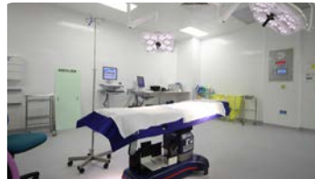
Kettering Maternity Theatres £1.4m (M&E)
