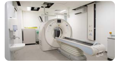
Leicester Emergency Department – CT Scanner £0.9m (M&E)
